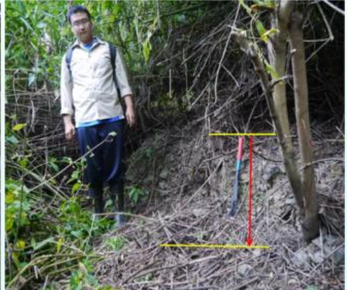
D: Extension crack
